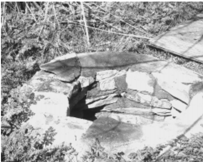
This open cesspool is a serious potential safety hazard.
