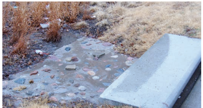
Figure 4. Debris in a bioswale at a curb inlet.
