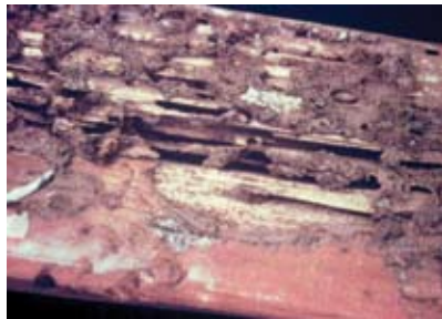
Figure 5 – Mud-filled joints in wood
