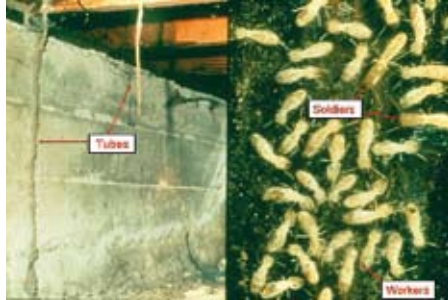
Figure 5 – Termites and Termite Tubes
